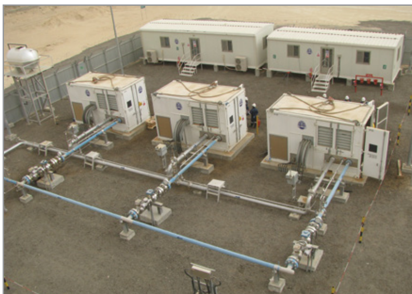
High Pressure Water Injection Pumps.
